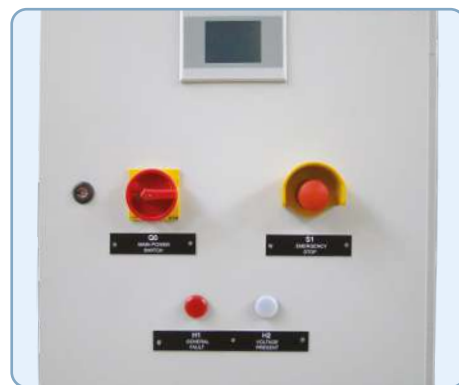
Electrical control panel
